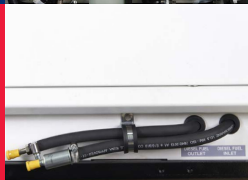
Input/Output fuel pipe
