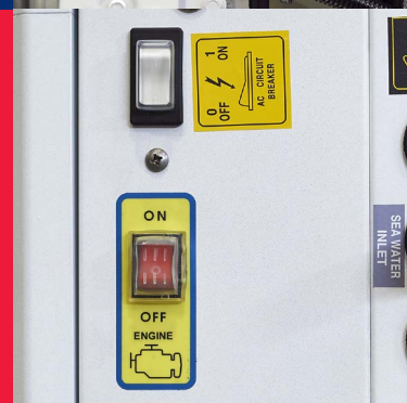
Main circuit breaker
