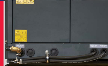
Input/Output fuel pipe
