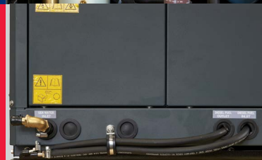
Input/Output fuel pipe
