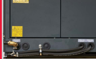
Input/Output fuel pipe
